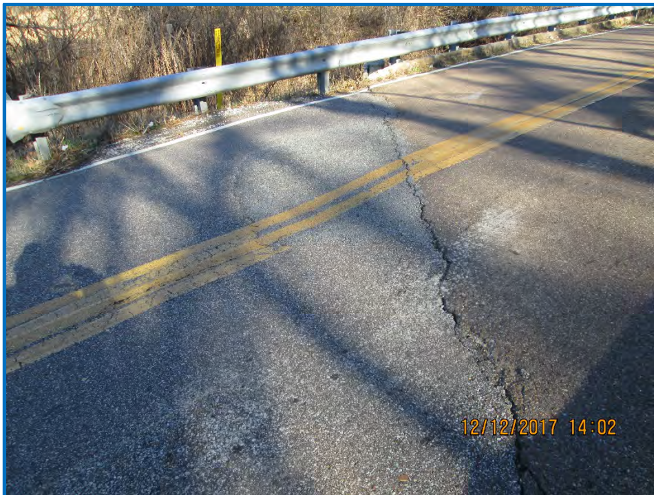
Pavement failure at west end of bridge
